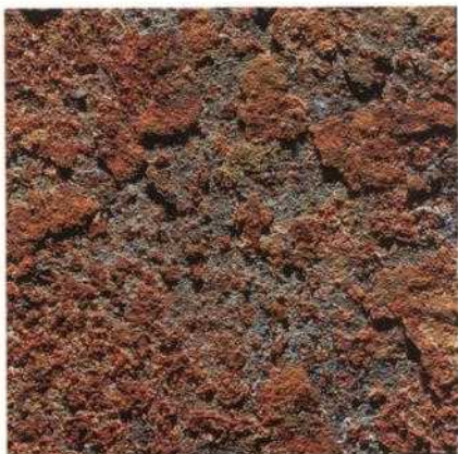
INITIAL CONDITION D
