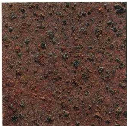
INITIAL CONDITION D
